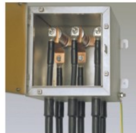
Link box installed with cross bonding cables
